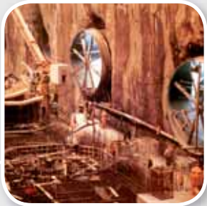
Xiaolangdi underground power plant, China
